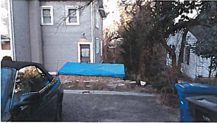
Street view of unfinished shed, prior to requested repositioning.
