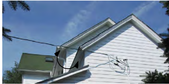
MATCHING CORNICE AND EAVE DETAIL (EXISTING TO BE RESTORED IN NEW LOCATION OR REPLICATED)
