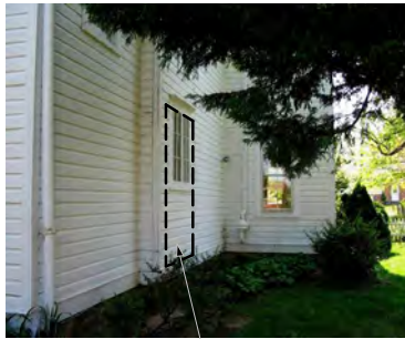
North Side Door Location @ Window Location (note window cap detail to be replicated) (Above)
