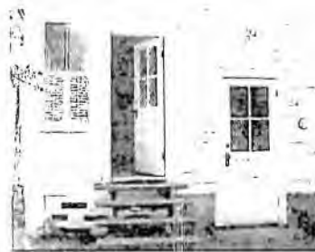
SIDE STEPS (To Be Removed )
