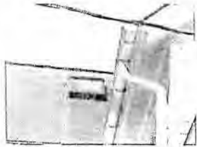
One of the Existing VELUX skylight on main roof (The New Skylight to match )
